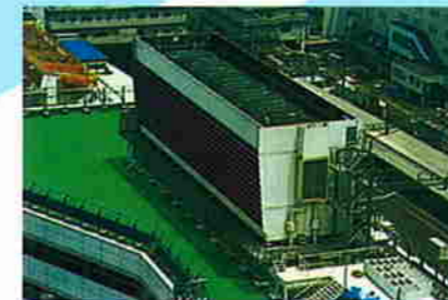
Crossflow type Cooling Tower for district cooling
