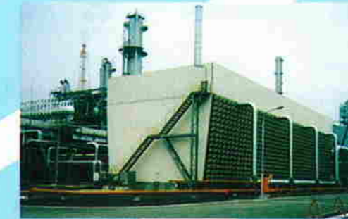
Crossflow type Cooling Tower for industrial process cooling
